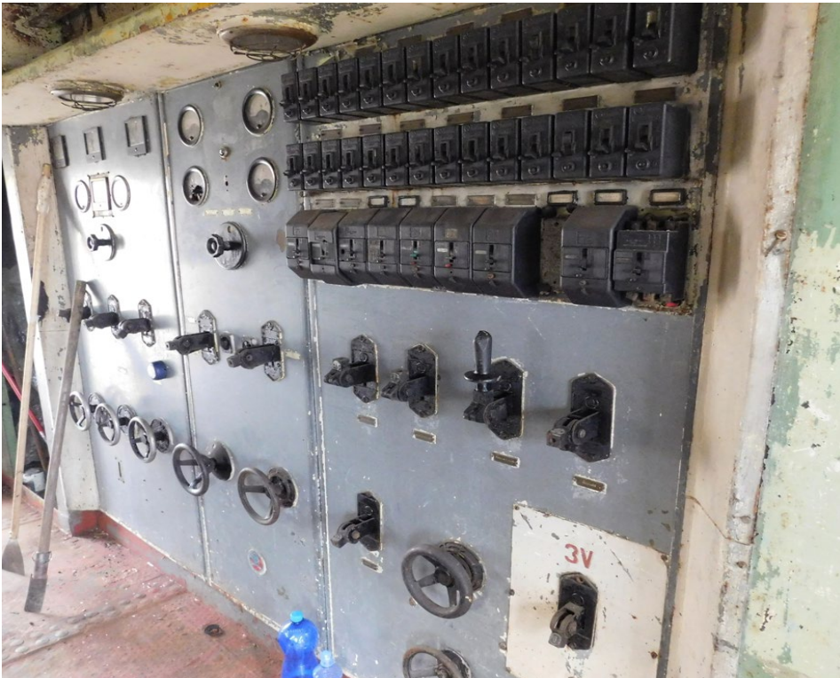
Engine room (current state before restoration) Source: Archive of STM-MD in Bratislava
