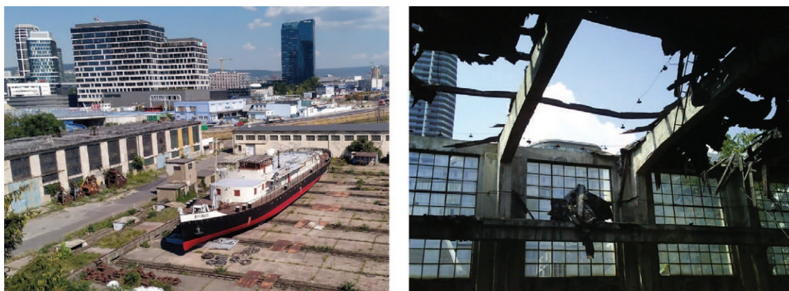
Fig. 2 (left) Shipping Hall with the ship elevator, on which is located the Tugboat ŠTUREC, photo: august 2022 © M. Goduš and (right) degraded roof of the Shipping Hall, photo: august 2023 © J. Mandl
